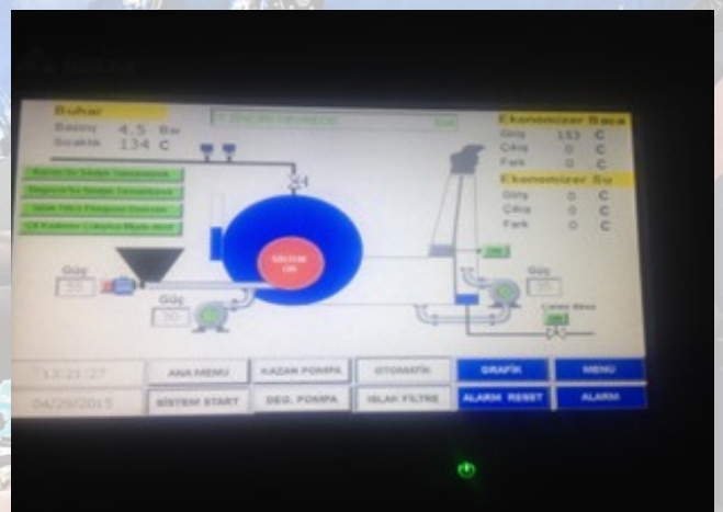
PLC and Automation Panel
