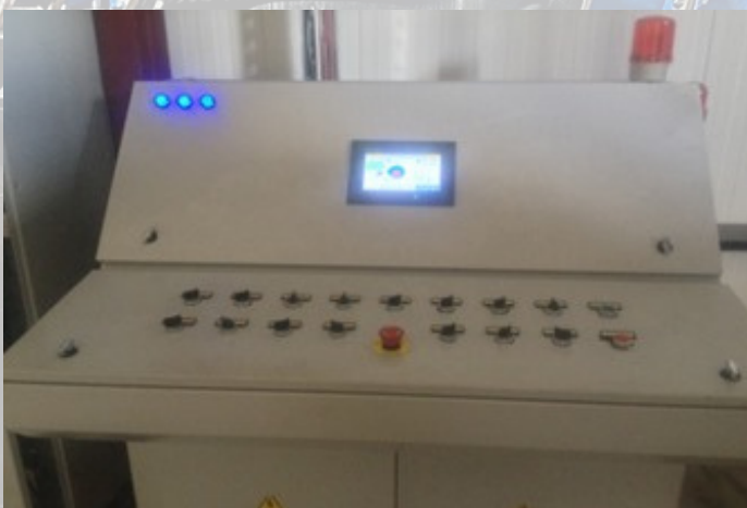
Piano Type Electrical Panel and Control System
